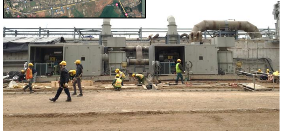
Project : Nghi Sohn Refinery Project, Vietnam Service : Desulfurization Oxidation Air Blower
