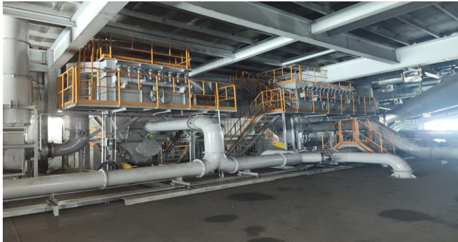
GS Power Tripper Room
