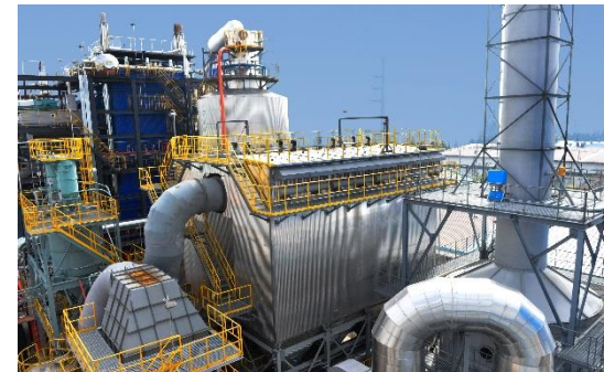
Bag Filter Facilities
