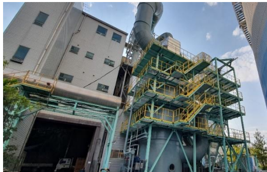
DS E&E Scrubber Facilities
