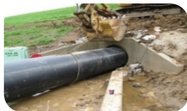
Waster Water Treatment
